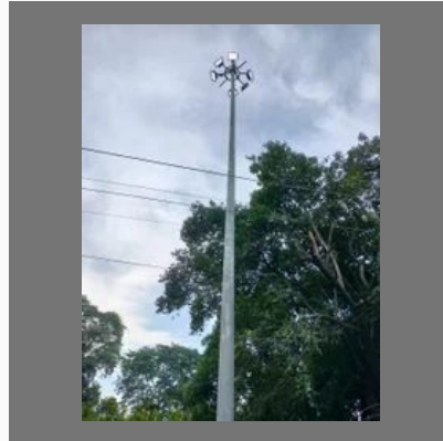
20 meters Led High Mast Lighting System
