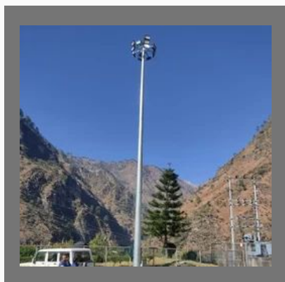
Mobile Lighting Tower
