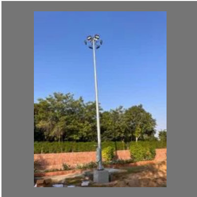
High Mast Lighting
