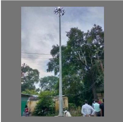
High Mast Lighting Pole
